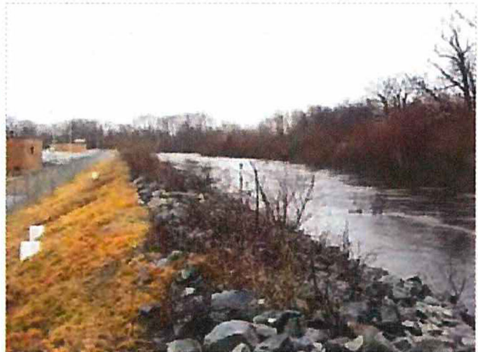
This levee, which protects the Warwick WWTF, was breached on March 30, 2010, flooding the treatment plant area
