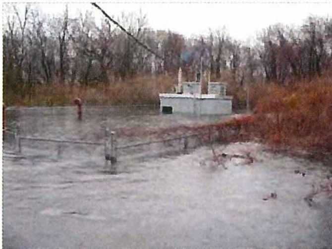
Warwick Sewer Authority's Knight Street pump station can operate underwater
